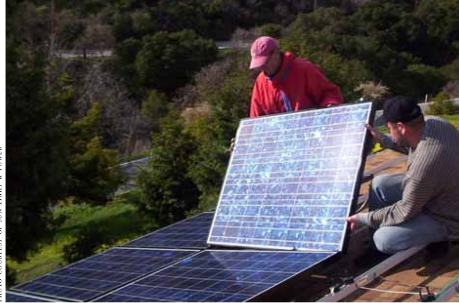
PHOTO COURTESY OF SUN LIGHT & POWER
